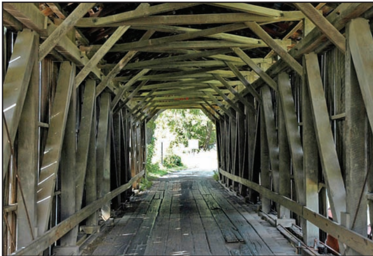
The Foraker Bridge in Monroe County is a good example of the Multiple Kingpost timber frame construction.
